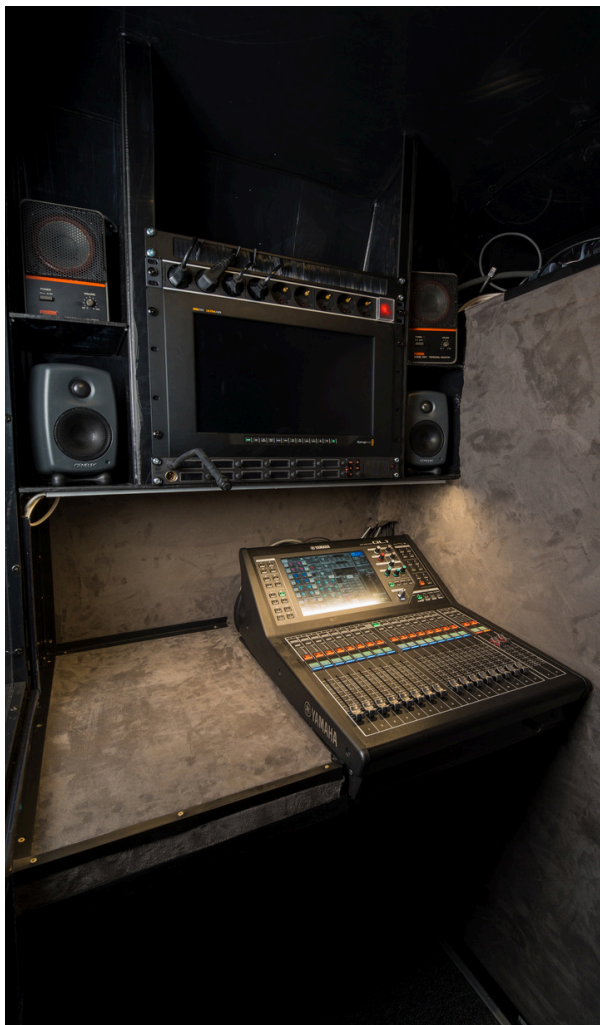
Sound engineer room
